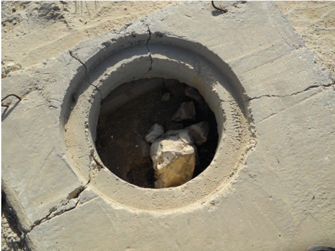
Figure 4a. The harabeh , a pit for rainwater, blocked-up by JNF, December 5, 2016.
